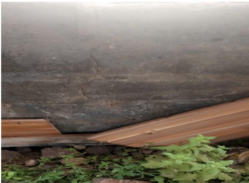
Figure 3b: Photographs of cracked building walls
