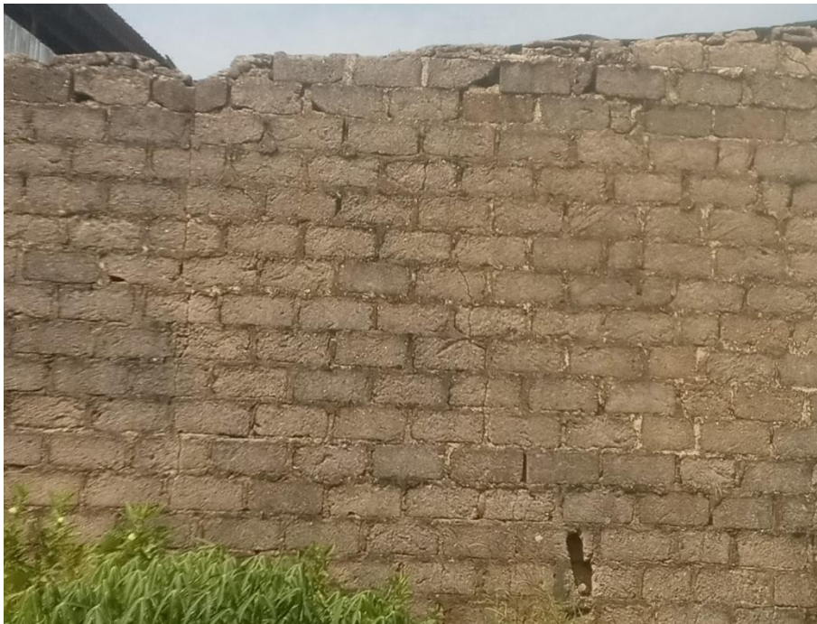
Figure 3a: Photographs of cracked building walls
